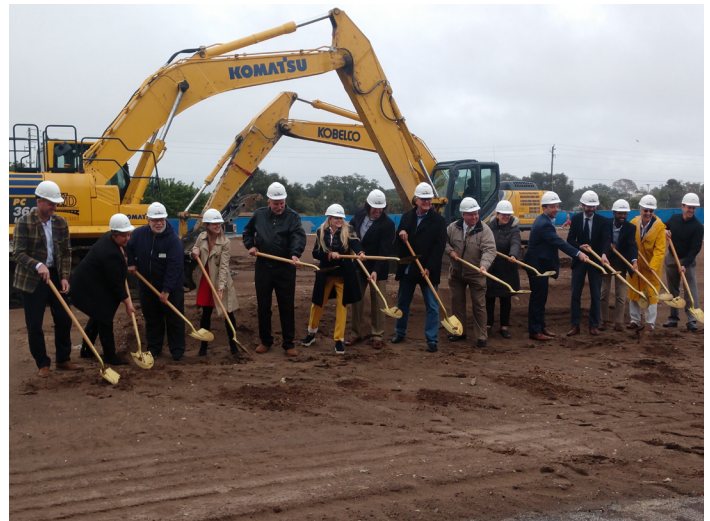
Hutton Group broke ground in early 2020 on their Rockledge Flats apartment project
