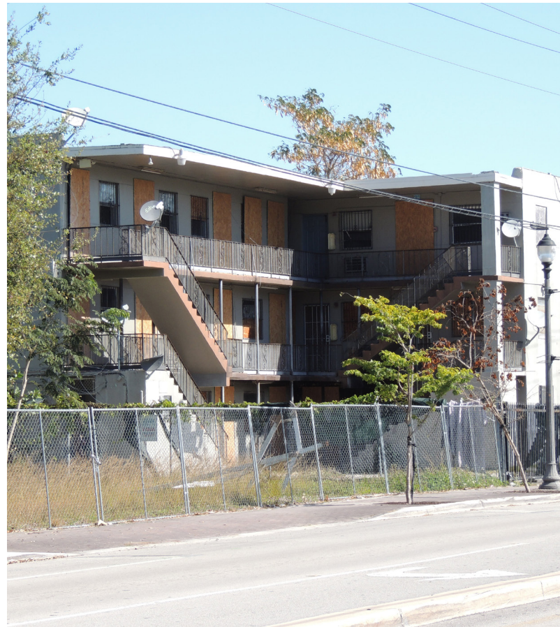
Image: A building in disrepair in the West Grove neighborhood. (Source: Plusurbia Design, 2021)
