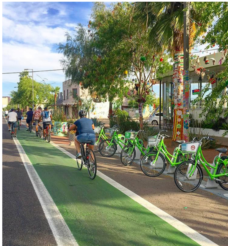
Image: Newly constructed bicycle lanes. (Source: Making Way for Complete Streets, wginc.com, 2020)
