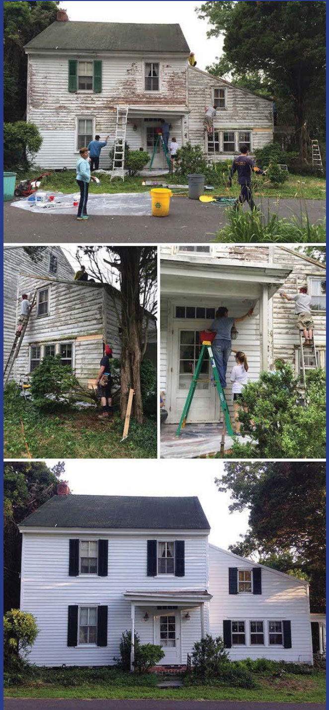
Image: Before, during, and after images for a home repair. (Source: Go Humans News)
